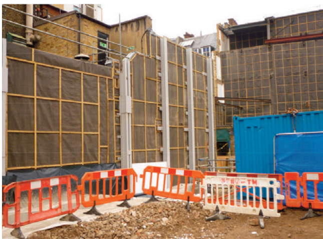
These 2 photographs show the site post-demolition with the temporary steels and weatherproofing fixed to the party wall
