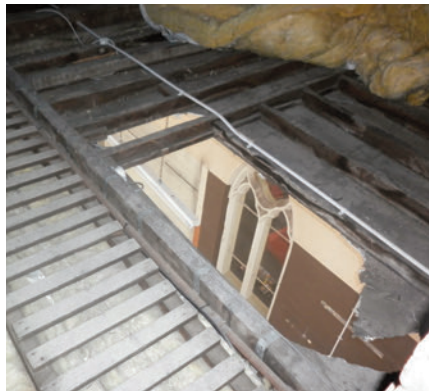
The hole caused by the individual's fall
