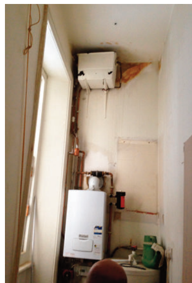
Advising the landlord and their solicitors on proposed alterations to a flat internal gas supply
