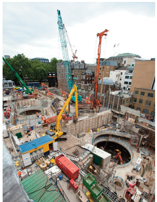
Both temporary access shafts can be seen, but eventually the whole site will be excavated to form the station box
