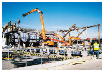
2004 Burnt out warehouse, Essex
