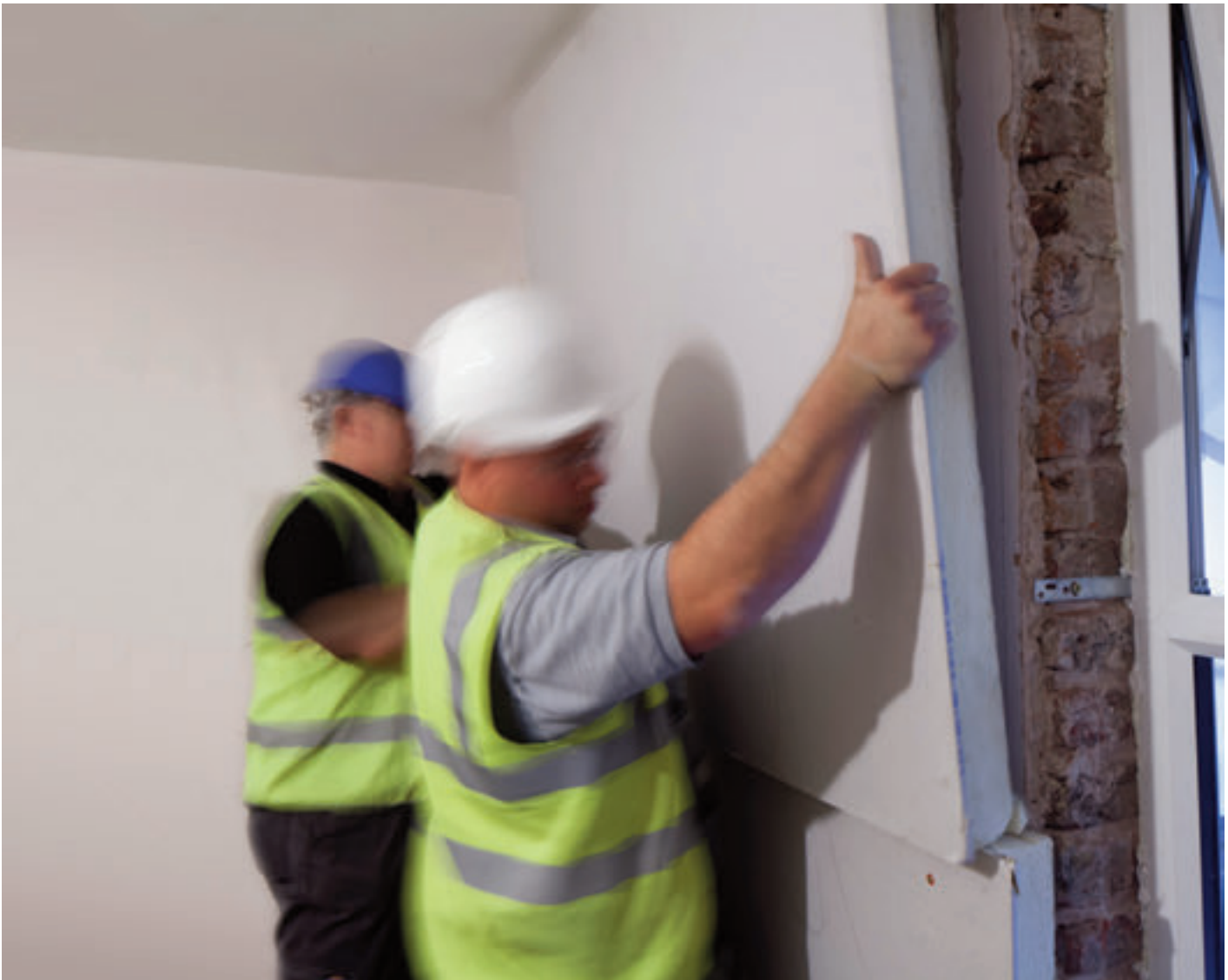
Fir for purpose: Installers fit Gyproc Thermaline PIR to internally plastered brick walls
