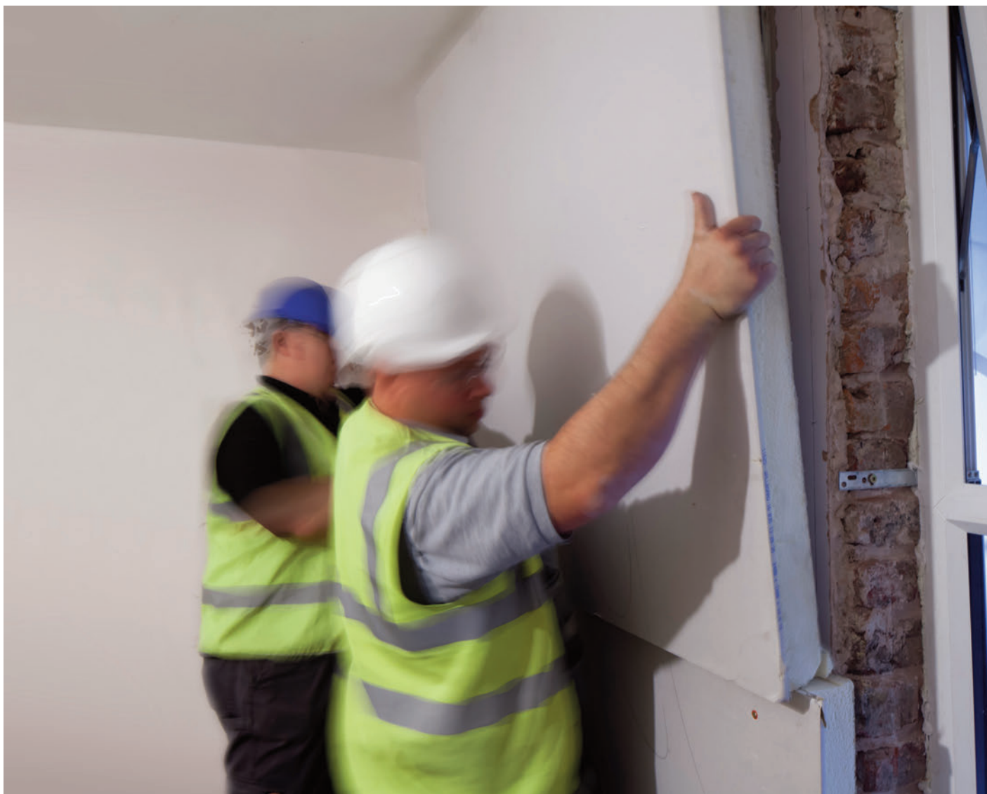
Fir for purpose: Installers fit Gyproc Thermaline PIR to internally plastered brick walls
