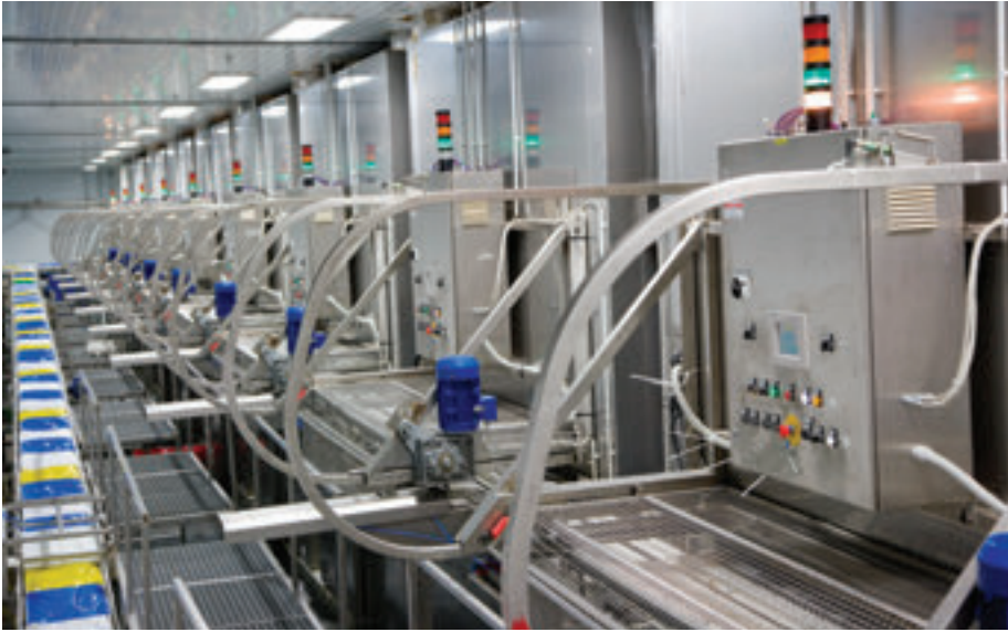
A line of hi-tech freezers from Skaginn and affiliates at a modern pelagic processing plant in Eastern Iceland.
