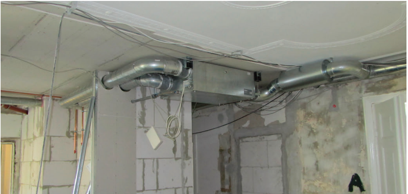
Here a decentralised HRV system from Ecovent / Øland is mounted in connection to urban renewal at Gl. Kongevej in Copenhagen
