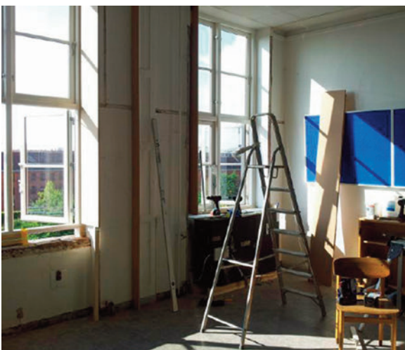
The window integrated heat recovery ventilation technology installed in a Copenhagen school as part of the Nordic Built project. Here each of 3 HRV units provides 200-250m 3 /h of air
