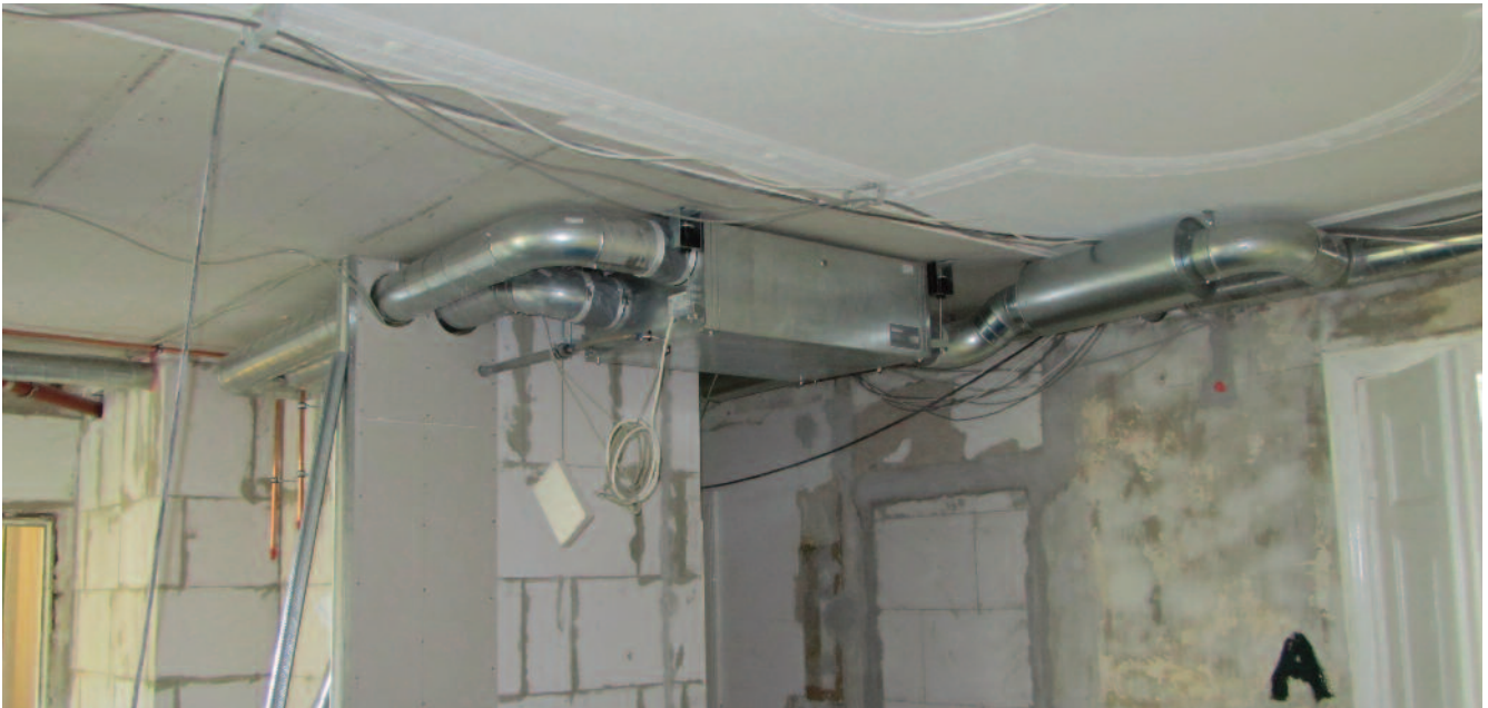
Here a decentralised HRV system from Ecovent / Øland is mounted in connection to urban renewal at Gl. Kongevej in Copenhagen
