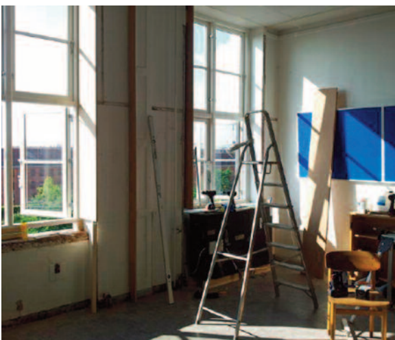
The window integrated heat recovery ventilation technology installed in a Copenhagen school as part of the Nordic Built project. Here each of 3 HRV units provides 200-250m 3 /h of air
