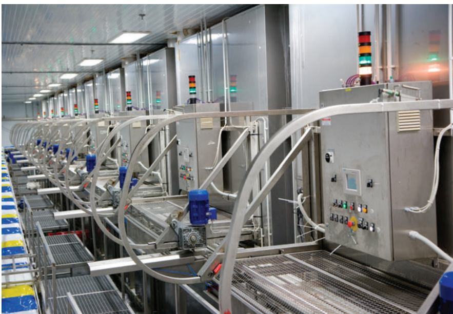
A line of hi-tech freezers from Skaginn and affiliates at a modern pelagic processing plant in Eastern Iceland.
