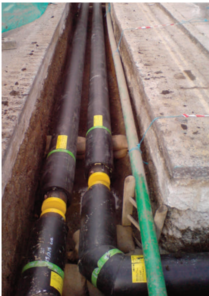
A relatively simple installation of district heating network in the highway. The pipes have been laid in place and are yet to be jointed
