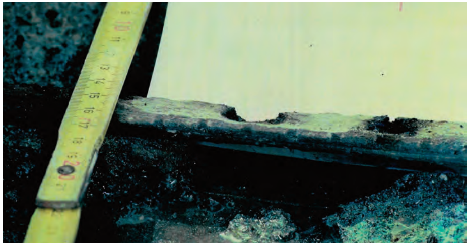
Figure 4: Localized chloride induced corrosion of the reinforcement showing that no rust is formed
