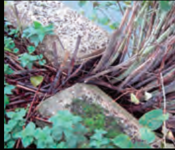
Example of Japanese Knotweed destroying a canal side kerb
