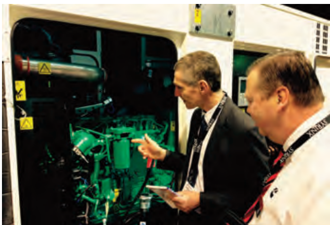
Malcolm Kent, left, discusses engine technology with Gary LaFine of Cummins Power Generation. Constant speed engines such as these will need to jump from Stage IIIA to Stage V in 2019.
