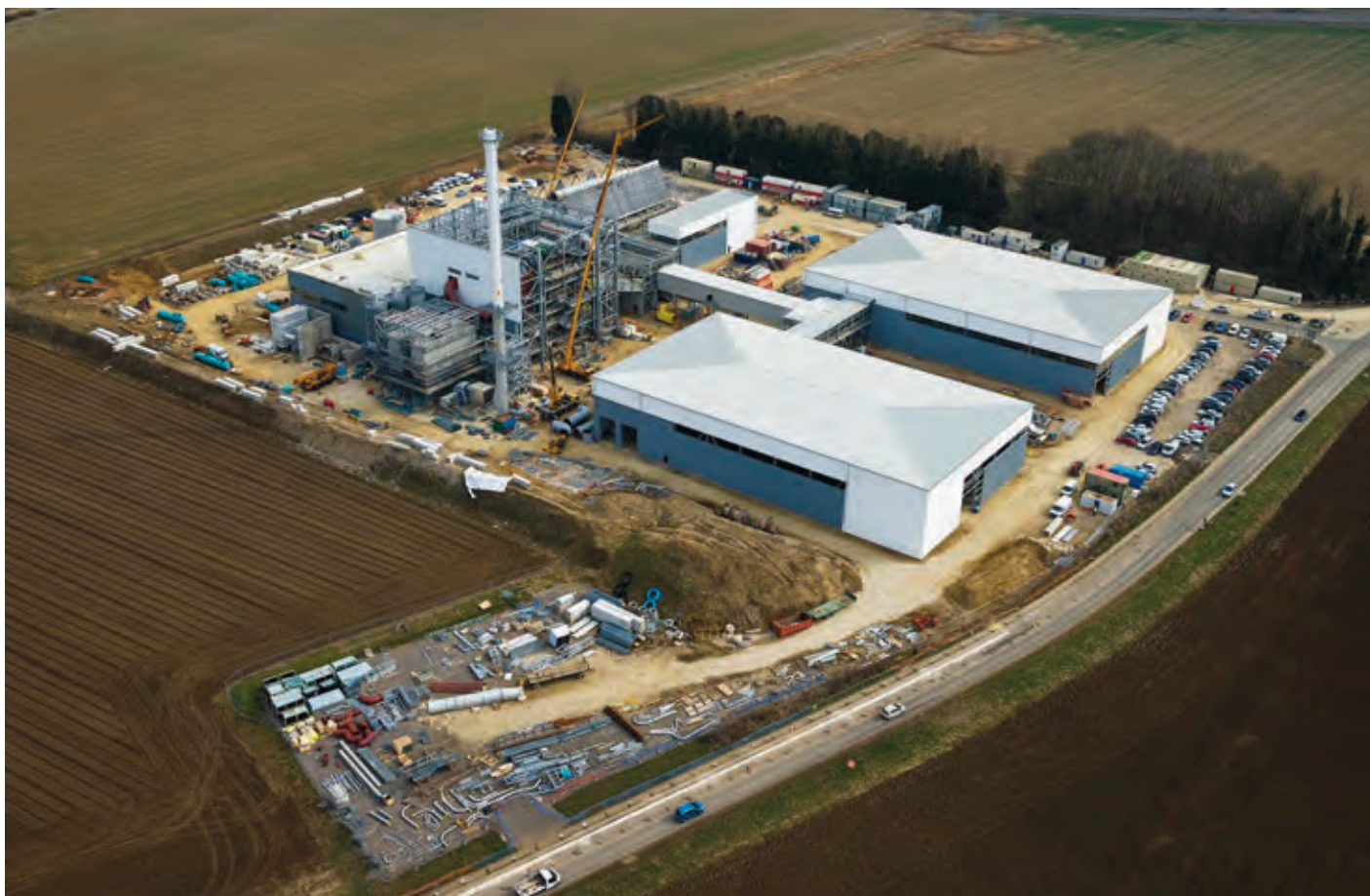
Image courtesy of Caunton Engineering Ltd
