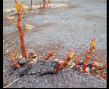
Example of Japanese Knotweed destroying a car park
