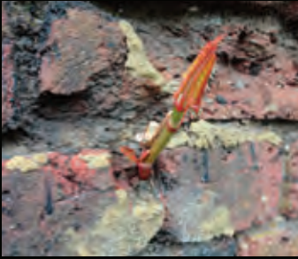
Example of Japanese Knotweed breaking through a brick wall
