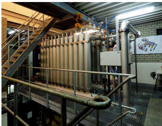
Figure 2. Picture of the ceramic membrane filtration demonstration plant at Vitens production location, Wierden, NL
