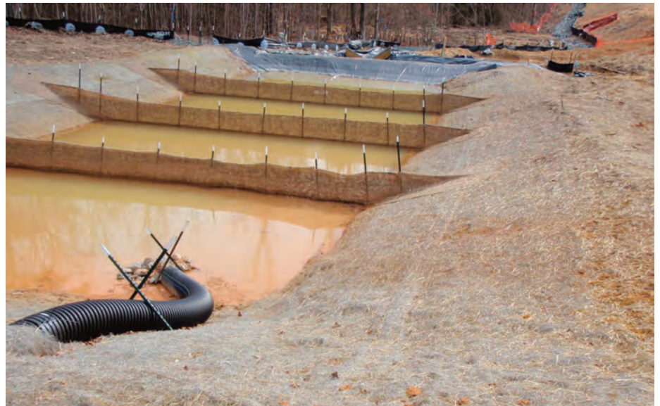
Example of a construction site sediment basin featuring a piped inlet, porous baffles, and a skimmer outlet
