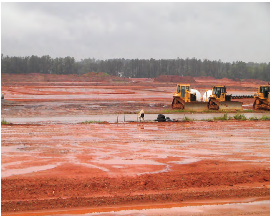
During construction projects, large amounts of soil may be exposed to erosion
