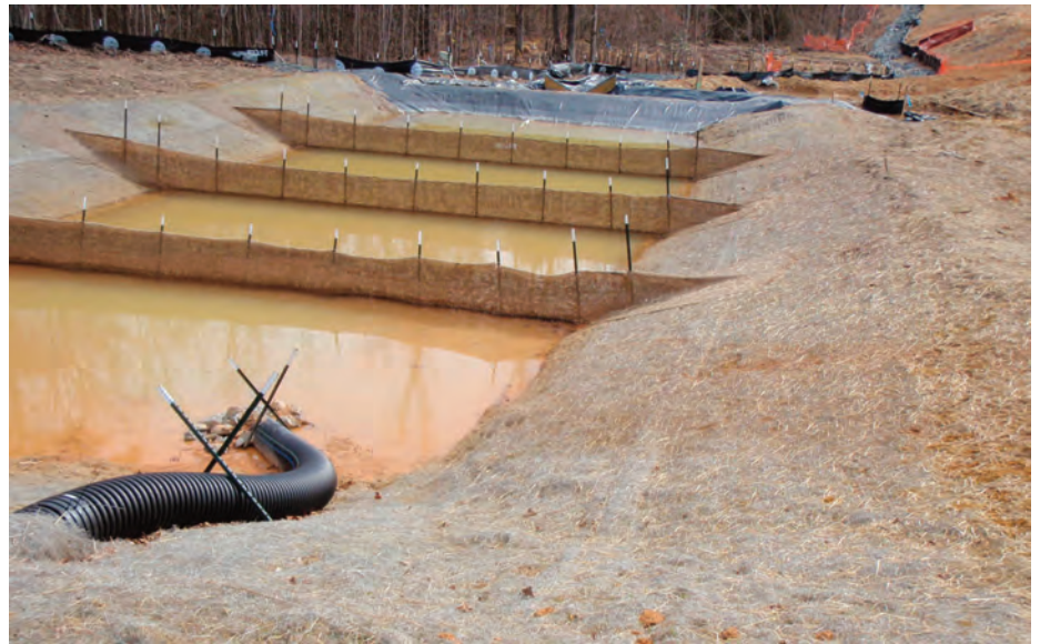
Example of a construction site sediment basin featuring a piped inlet, porous baffles, and a skimmer outlet
