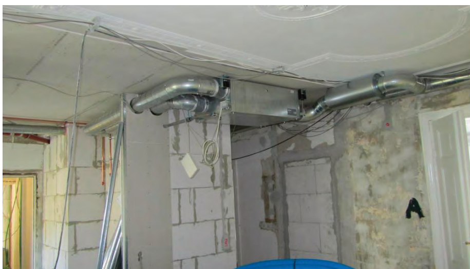
Here is shown an optimised decentralised HRV system from Ecovent / Øland mounted under the loft in connection to urban renewal at Gl. Kongevej in Copenhagen
