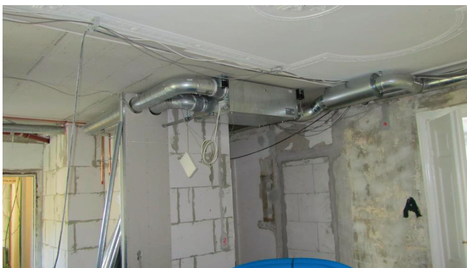
Here is shown an optimised decentralised HRV system from Ecovent / Øland mounted under the loft in connection to urban renewal at Gl. Kongevej in Copenhagen
