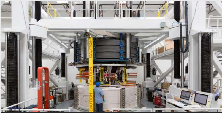
A segment of the colossal Central Solenoid magnet, "the beating heart of ITER," under fabrication at General Atomics near San Diego, California, USA.
