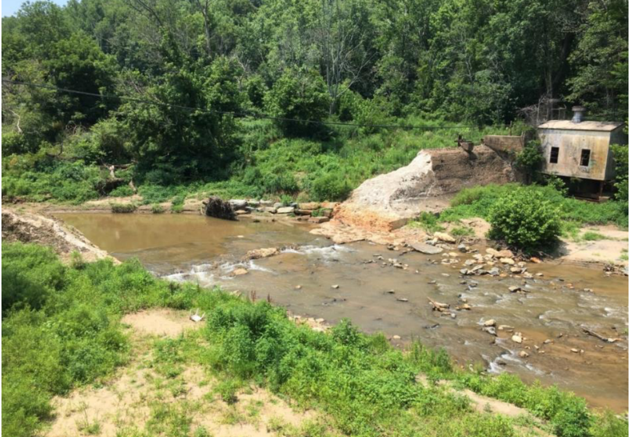
Figure 1 – Removal of a Low-Head Power Dam. The legacy sediments behind this structure have been distributed throughout the stream bed up to 50 km downstream.
